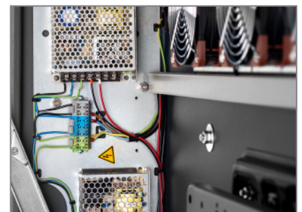
Cabling according to VDE guidelines
